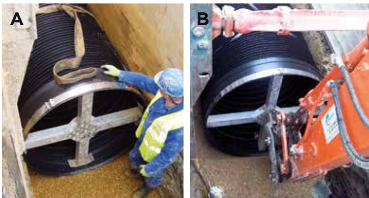
Figure 11: Image A - Aquaspira jointing frame. Image B - CSR pipe jointing utilising excavator arm.
