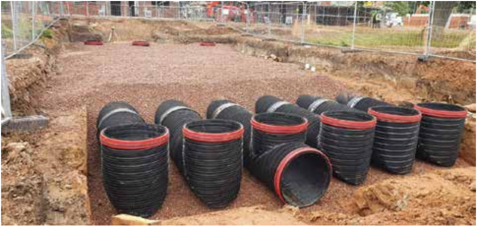
Figure 32: Picture of a multi-leg tank being backfilled evenly starting from the manifold.
